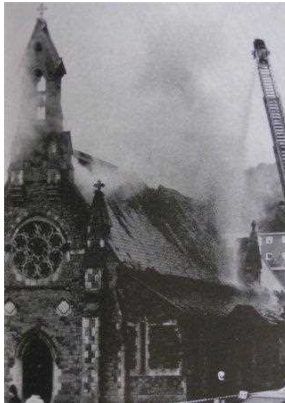
Another view of the tragic 1987 fire, showing the severe damage to the roof.
