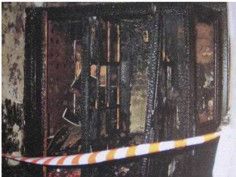
The remains of the Confessional where the arsonist started the 1987 fire in St Paul's Church
