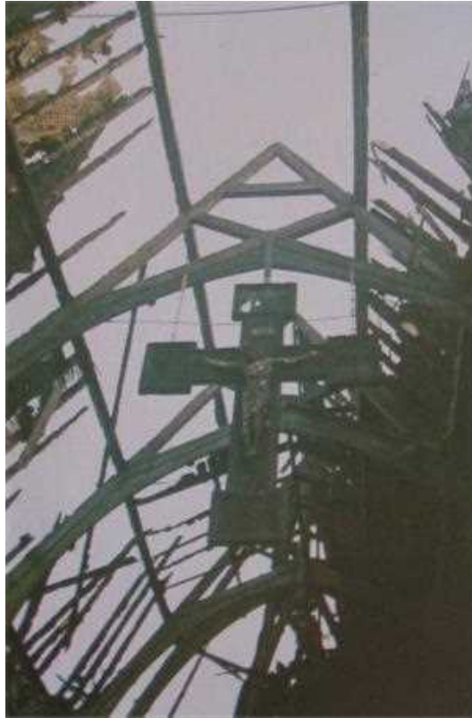
The desolation of the Cross: the once beautiful and now charred Crucifix hangs in stark desolation from the remains of the roof structure following the 1987 fire
