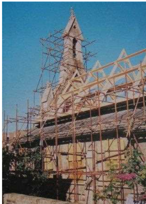
Resurrection: the new roof trusses and associated structure are in place as work advances on restoring the Church: 1988 July
